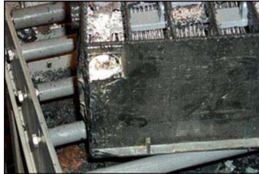
Corrosion --The positive terminal of this battery corroded so badly it became fused to the cable and broke. Note the internal corrosion on the strap and plates.
