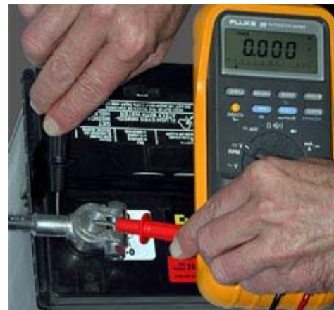
Checking for Poor Connection
